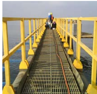
Gratings on Walkways Pultruded gratings on walkways of an oil rig, exhibits tremendous benefits in highly corrosive environment.
